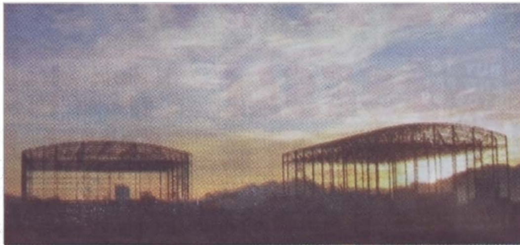
IN FRAME: The two giant steel skeletons of Studio One and 3 of the Cape Town Film Studios as seen from the corner of the N2 and Baden Powell Drive, near Faure.
